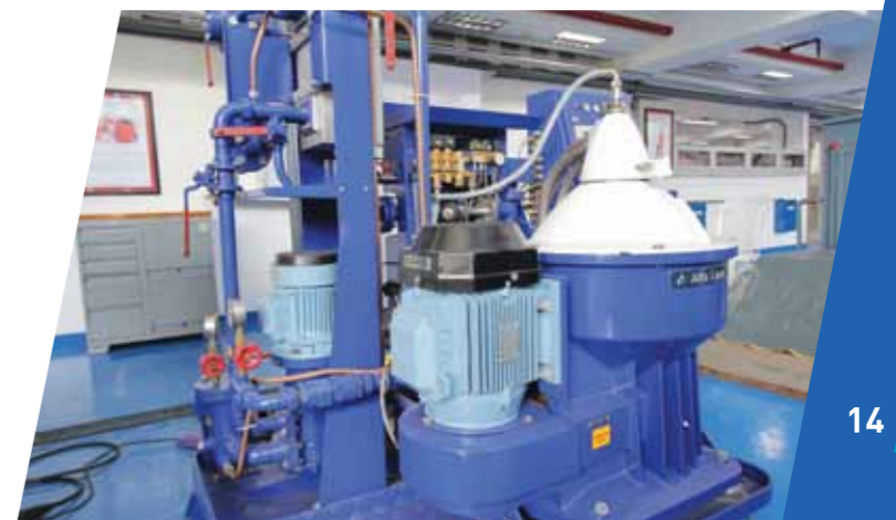
New Alfa Laval fuel management equipment at UMTC
